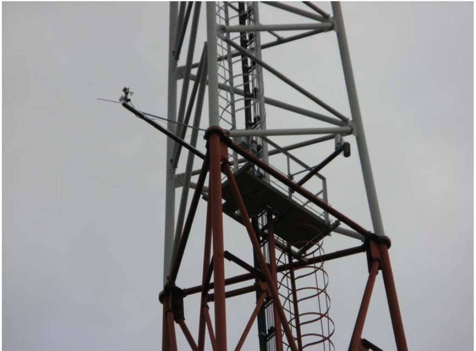
Figure 2 Overall view of placement weather station on cellular tower
