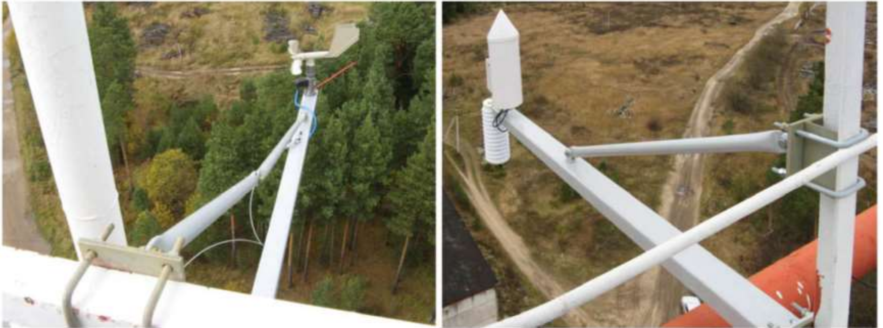
Figure 1 Wind speed and direction sensor, temperature and humidity sensor and precipitation sensor are placed on cellular communication tower
