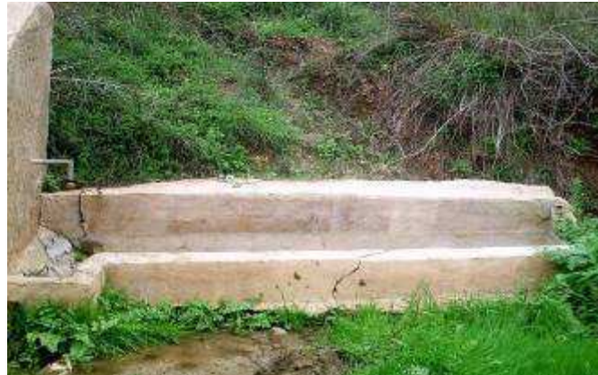
Photo 3: Damaged water place to be repaired
