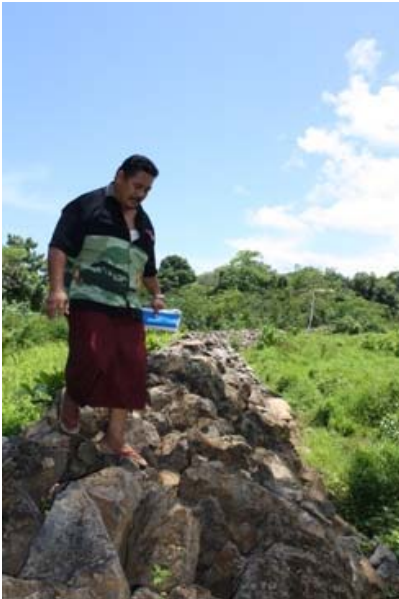
Figure 3: Tiuli Vao Foti, Salei'a CBA village committee member and a self-employed electrician, standing on the project site where a 200-metre retention wall was built and more than 200 trees were replanted along the stream against flooding and coastal erosion.
