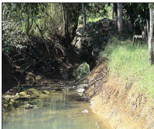
An eroded riverbank in the Bunkers Hill community. Climate change is likely to increase the intensity of storms in the area, raising the risk of flash flooding, exacerbating existing erosion problems, and threatening the croplands and infrastructure the community depends
