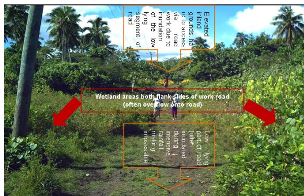
Work Road significantly affected by wetland flooding
