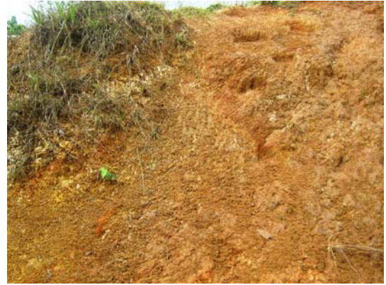
Soil erosion in Bellevue
