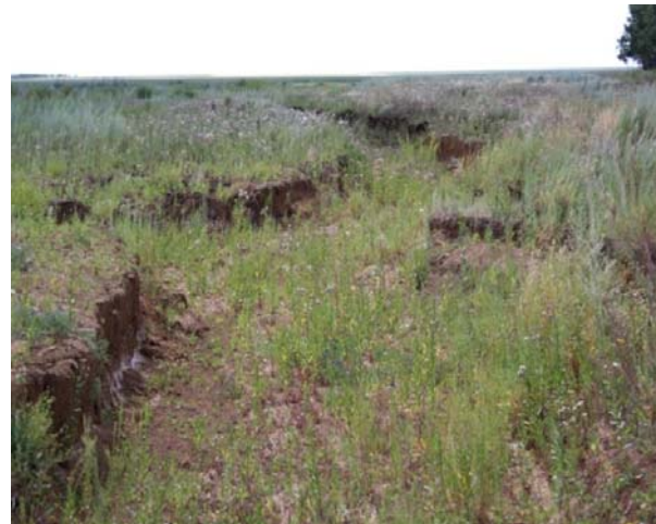
Severe erosion damage in the project area
