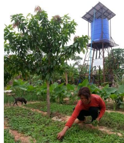
Solar pump station supplying water for vegetable gardening in Preah Vihear, Cambodia
