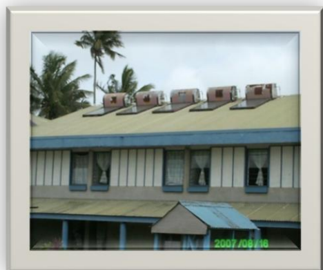
Photo 2.1: Solar thermal collectors as renewable energy sources in Tonga
