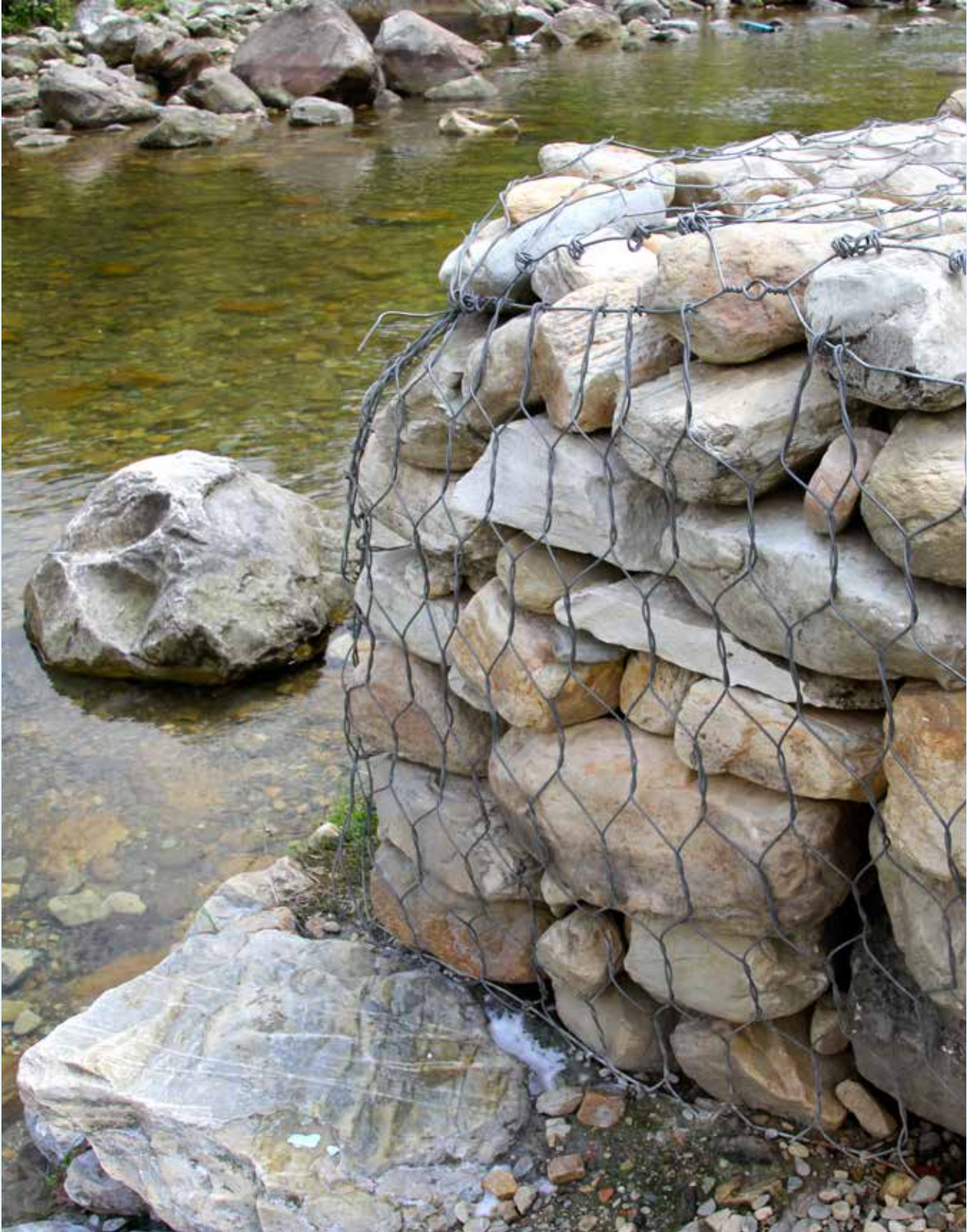
A GABION WALL CONSTRUCTED IN THE HARPAN RIVER, NEPAL, TO HELP PREVENT SILTATION AND RIVERBED EROSION. © Andrea Egan, UNDP
