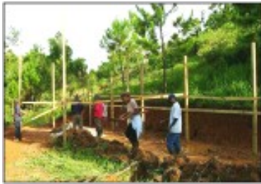
Community members participate in the construction of a greenhouse to be used for organic farming. Photo: JCDT for UNDP CBA
