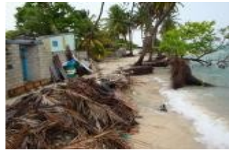
Houses vulnerable to coastal erosion on the island of K. Thullushdoo Photo: ICCRIP project document
