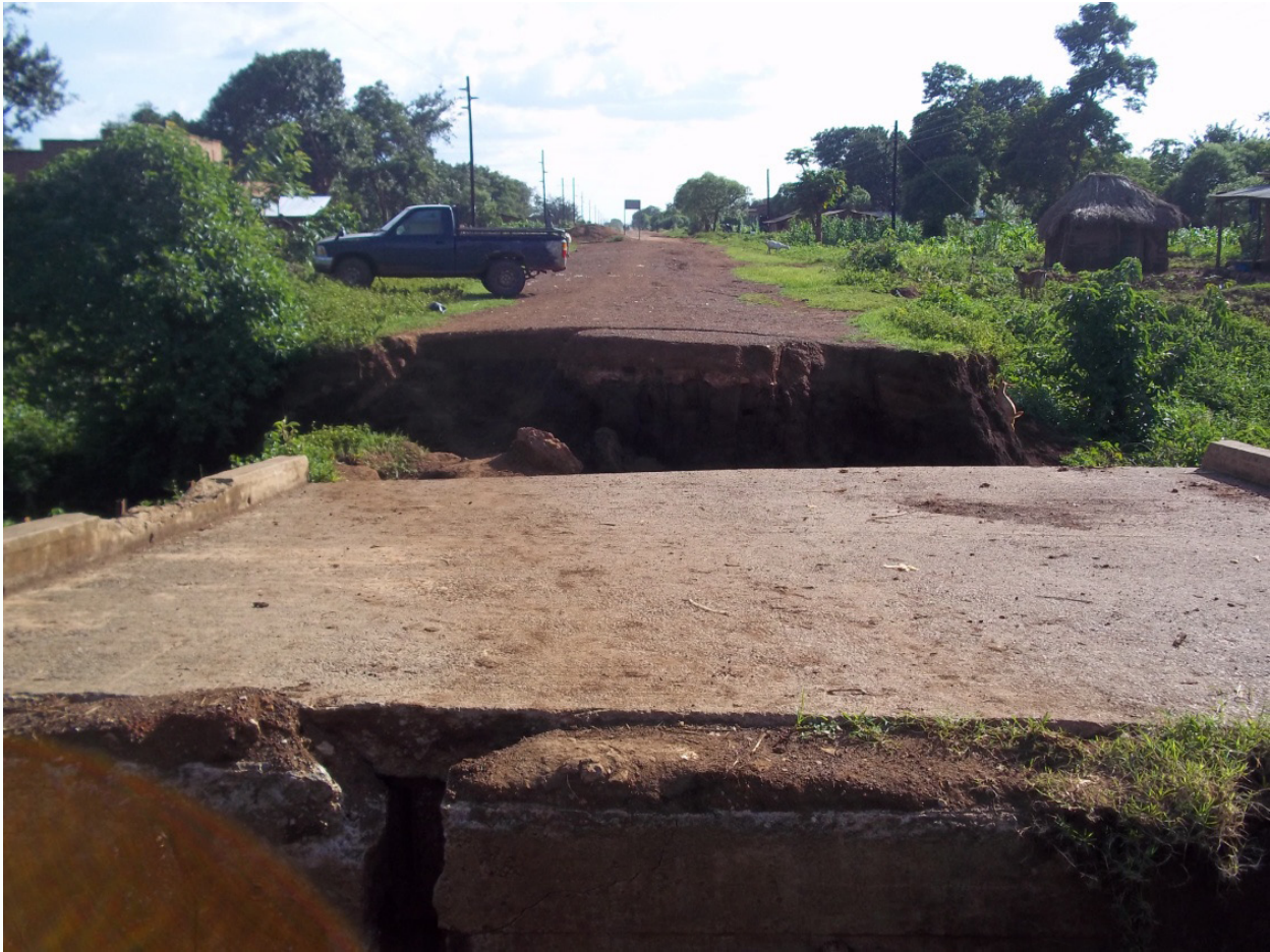
Plate 4.2. Damage to infrastructure such as roads (above: main Mbale – Nakapiripirit road) is common during the rainy season. Health and sanitation are among the elements of people’s lives that are most sensitive to flooding. As such,
