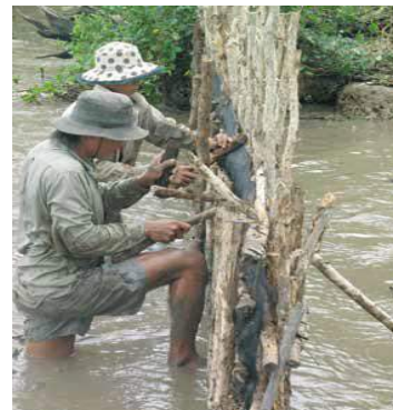
(b) Silt trap fence
