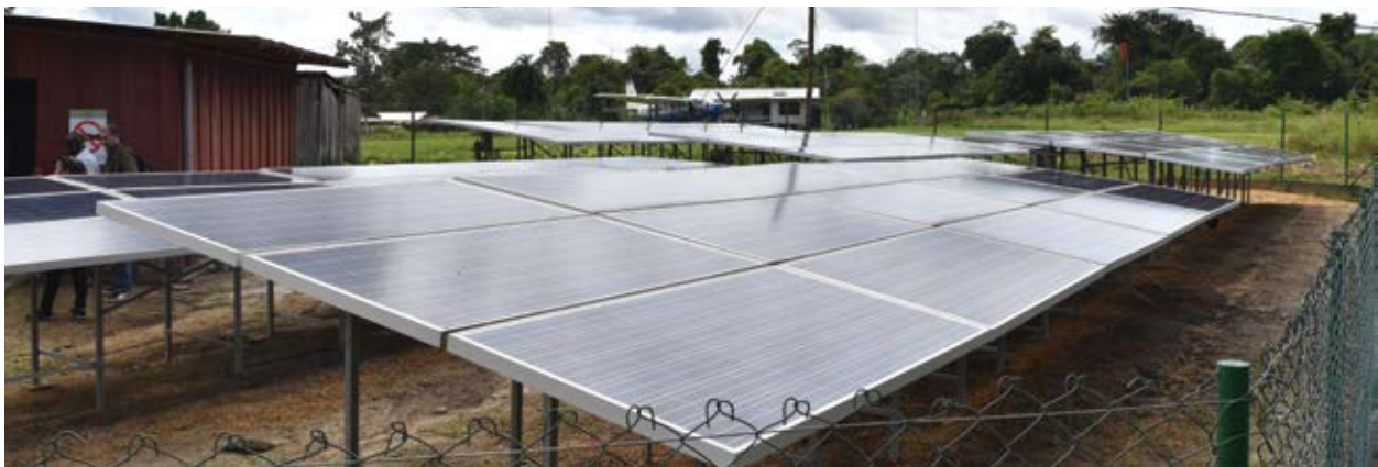
Solar PV system installed in Pelelu Tepu
