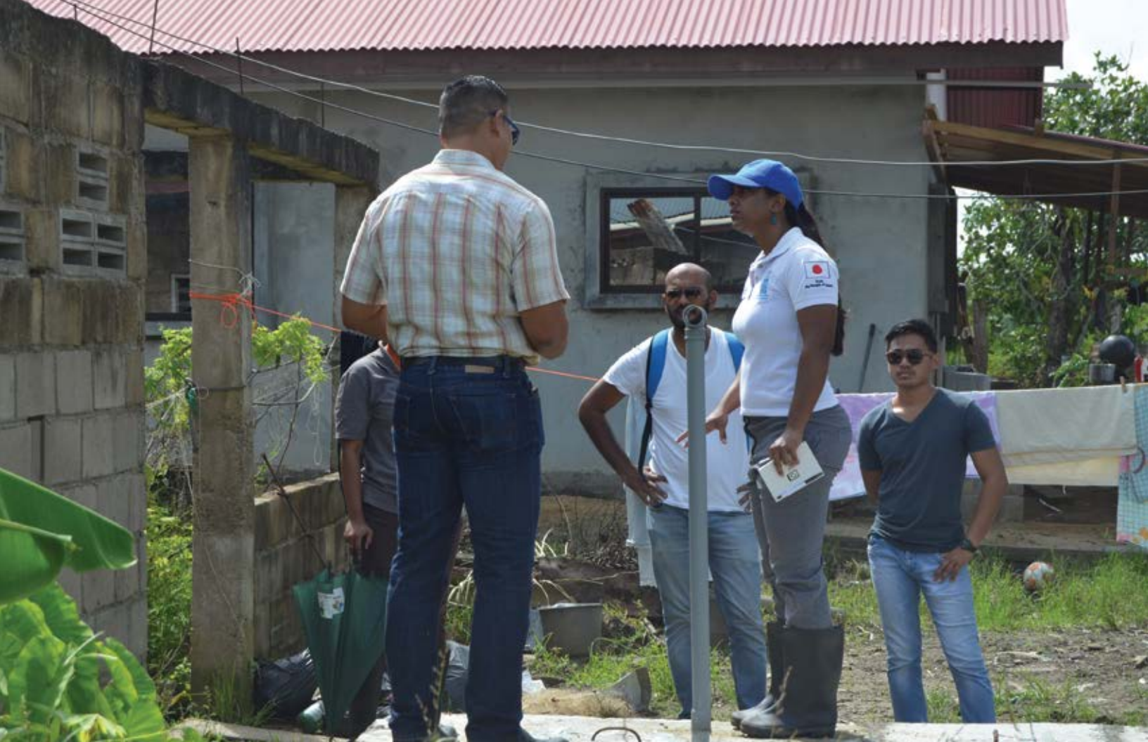
The project team stands on a newly installed septic system, while discussing the project's progress
