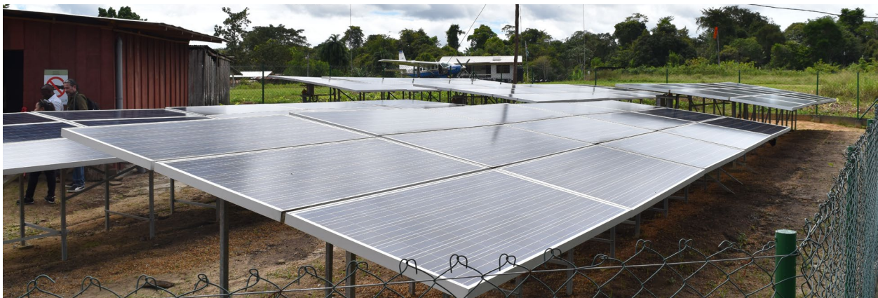
Solar PV system installed in Pelelu Tepu
