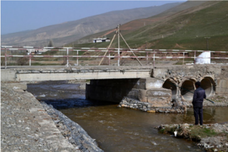
Flood impacts on infrastructure. Kyrgyzstan (Photo: UNDP)
