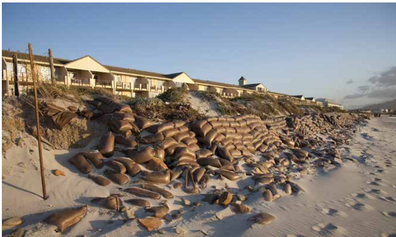
Coastal erosion and inefficient erosion reduction measures at Cape Town, South Africa. © 2009 SEI/Sean Wilson
